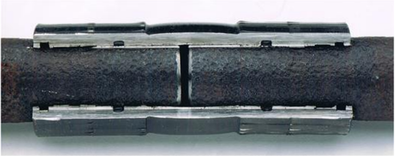
3/4" NPS Pipe-pitted due to years of exposure, Performed 6000 PSI Hydrostatic Proof Test and 1000 PSI Nitrogen Leak Test- No LEAKAGE DETECTED
